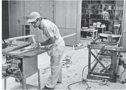
A construction worker putting the finishing touches on the Nitze Building in time for the October 1963 convocation
